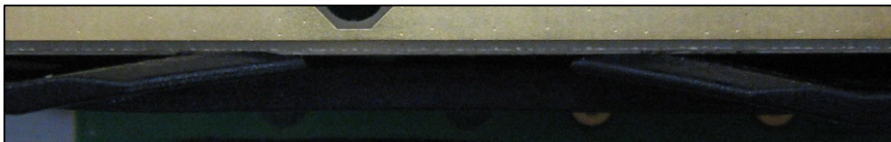
Plastic hooks: wrong installation
