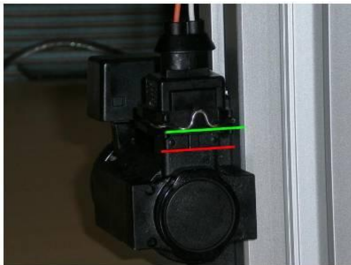
Figure 12: First of the possible assembly faults: plug completely connected.
