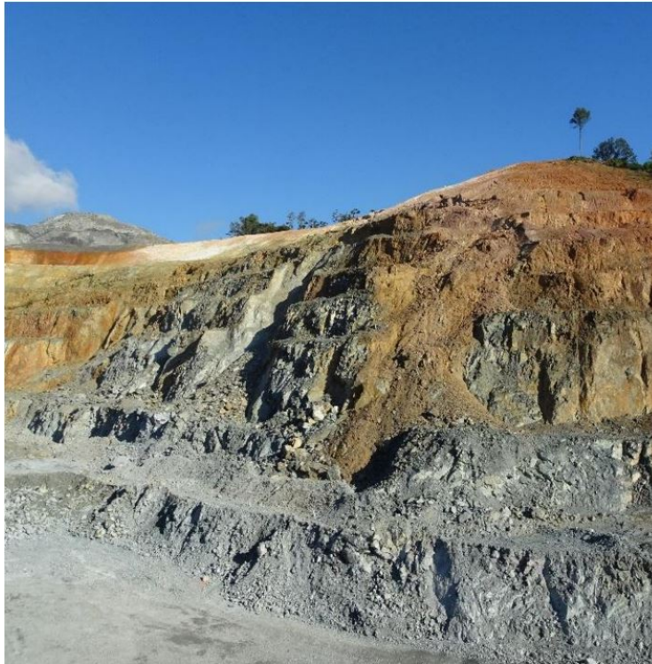
Figure 32: Photograph of Cumba Failure (Looking North-West, October 2019). Taken from: Bar et al. (2023)
