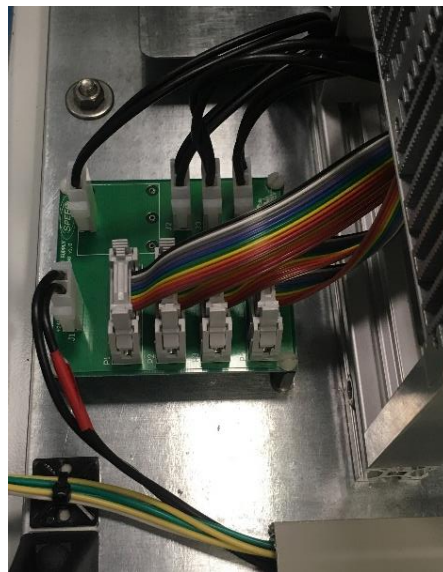
Chapter 1, Figure 36 - This electronic board is used to feed the four drivers and the four fans. The 24 V power is injected by the two pins terminal with the red sign; the white ten pin terminals feed the drivers while the white two pin terminal with completely black cables feed the fans. From a global point of view this board simplify the cables systems.
