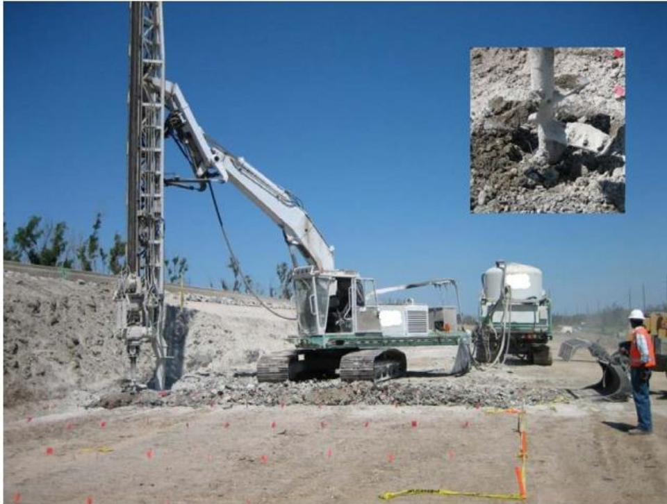
Figure 1.18. Deep mixing by the dry method; insert shows blades of mixing tool, with a port for binder delivery on the shaft (Schaefer et al., 2017a)
