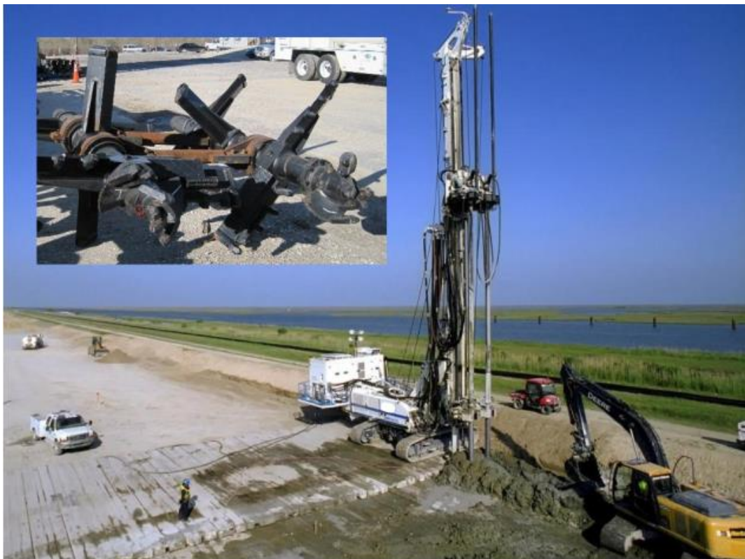
Figure 1.17. Deep mixing by the wet method; insert shows double axis mixing tool(Schaefer et al., 2017a)
