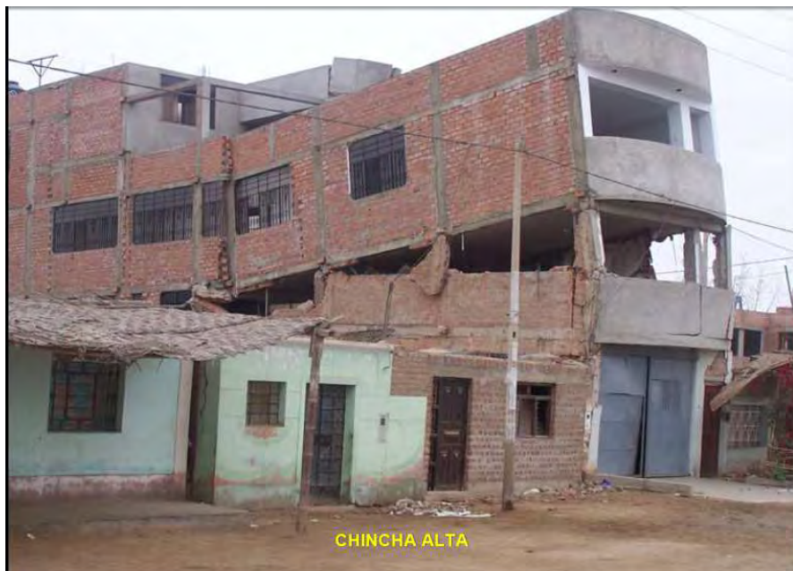
Fig. 3.13 – Partial emptying of several walls that cause the collapse of the second floor
