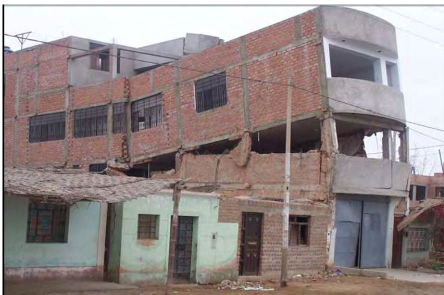
Fig. I.2 – Informal house condition after a seismic event
