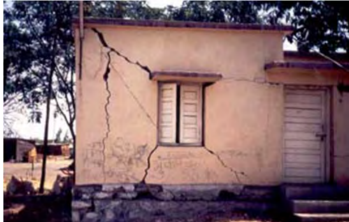
Fig. 1.8- Shear cracks in an unreinforced brick masonry building from the 1993 Killari earthquake
