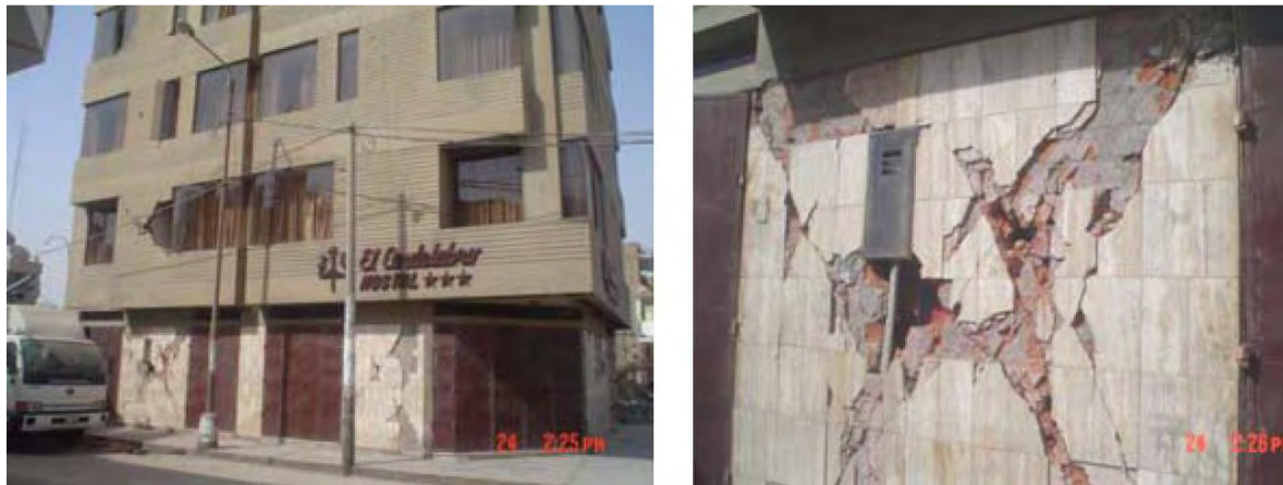
Fig. 3.12 – Insufficient shear strength of brick wall
