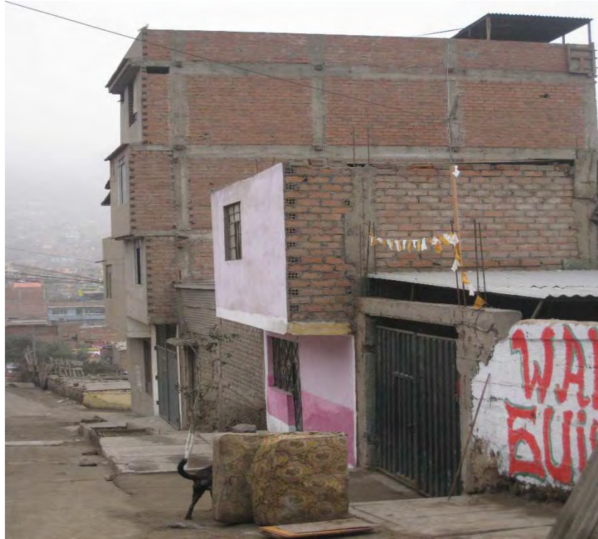
Fig. 3.4 – Discontinuity between first and second floor
