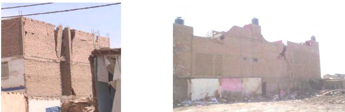
Fig. 3.8 – Wall failures due the absence of rigid diaphragm
