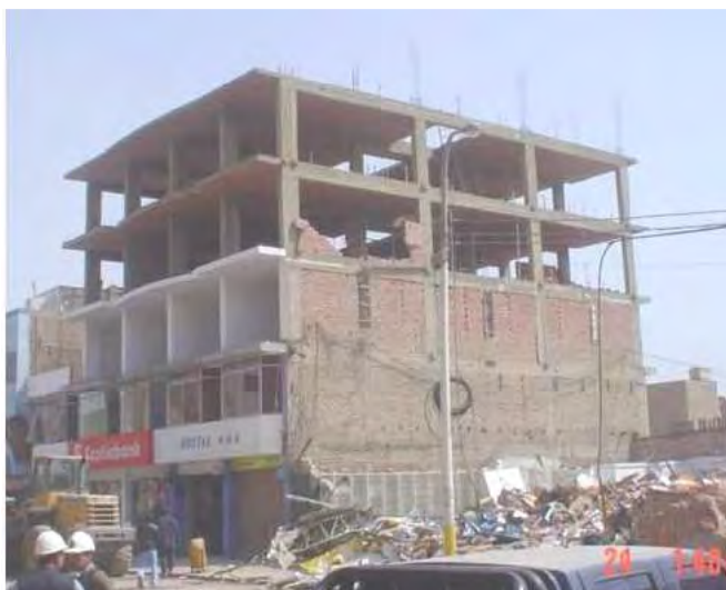
Fig. 3.10 – Lack of joint between columns and walls in the upper storeys
