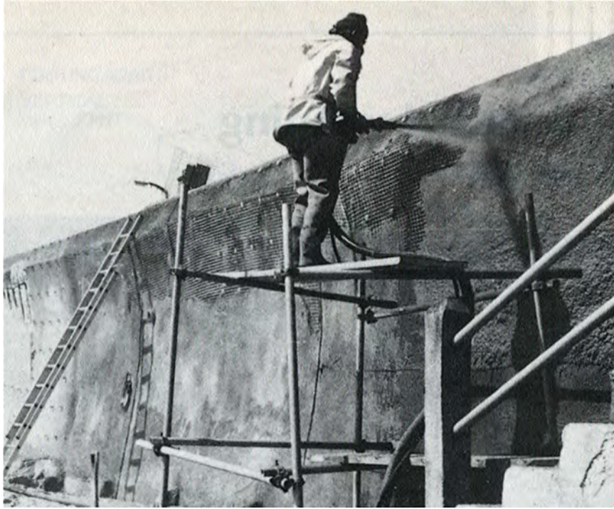
Fig. 1.30 - Polymer grid used for seawall repair is attached to nylon coated fasteners embedded in the wall
