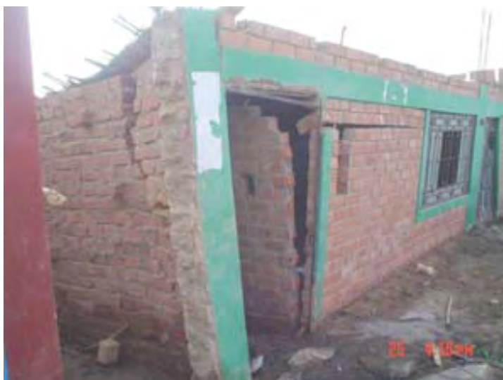
Fig. 3.11 – Partial collapse of brick masonry house due to the absence of confinement
