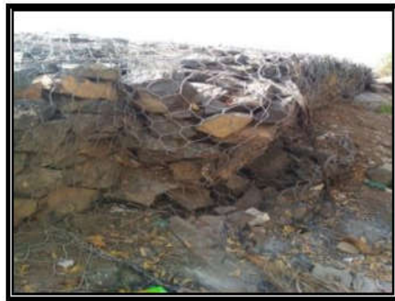
Figure 2.7. Bulging of Gabion mesh (Chikute & Sonar, 2019)
