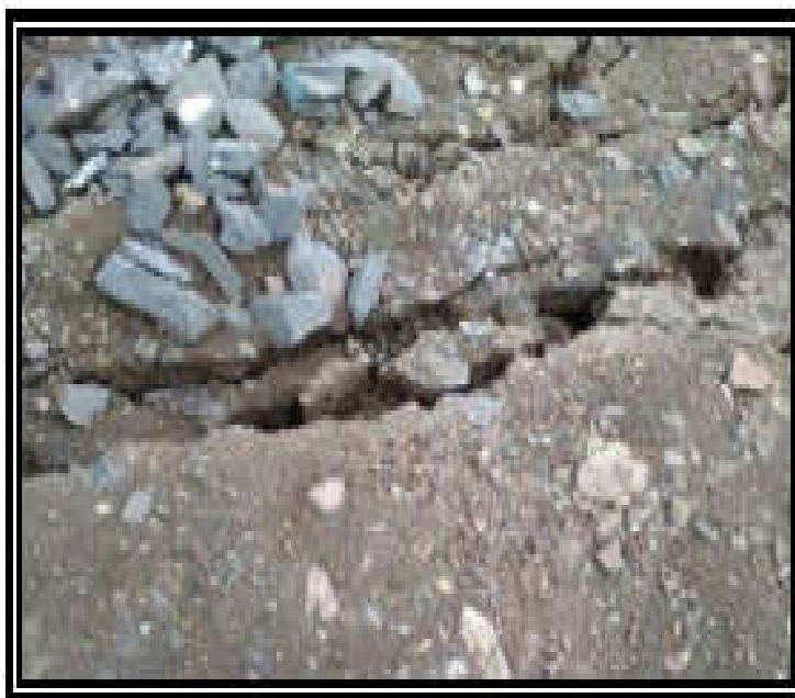
Figure 2.10. Crack in backfill (Chikute & Sonar, 2019)
