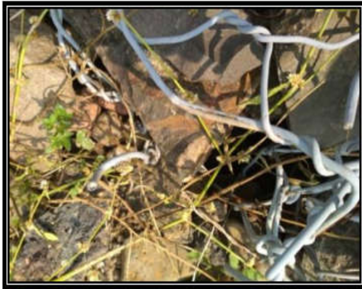
Figure 2.8. Corrosion of Gabion mesh (Chikute & Sonar, 2019)
