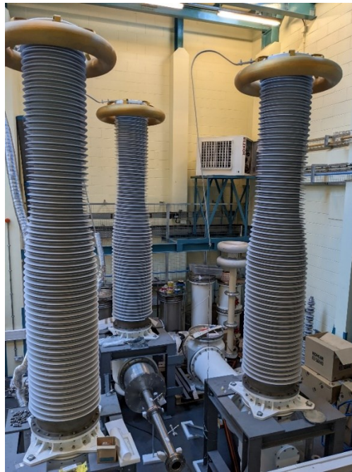
Figure 1.9. Barrel insulators used to isolate GILs at the Advanced High Voltage Engineering Research Centre situated in Cardiff University.
