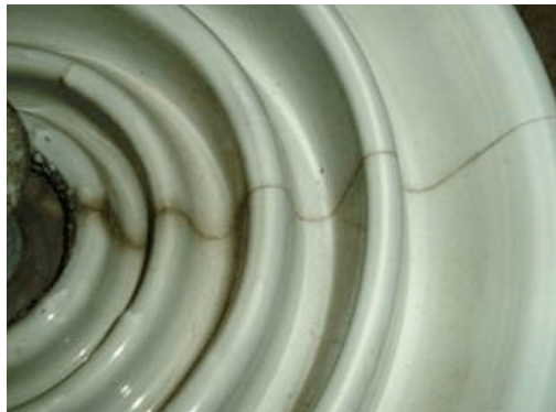
Figure 1.3. Effects of radial cracking in a porcelain insulator [3].
