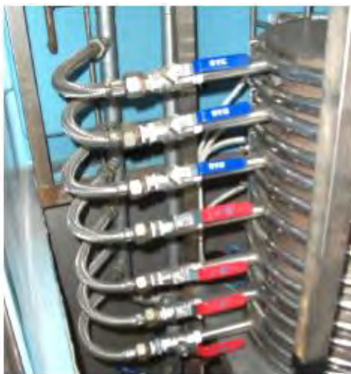
Figure 2.4. View of the cooling air distribution system to each section of the reactor
