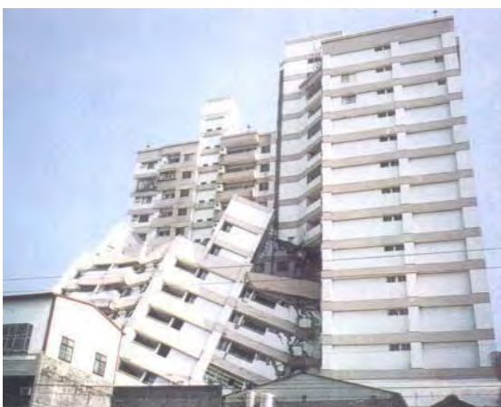
Figure 2.1 Example of the whole structure collapsed
