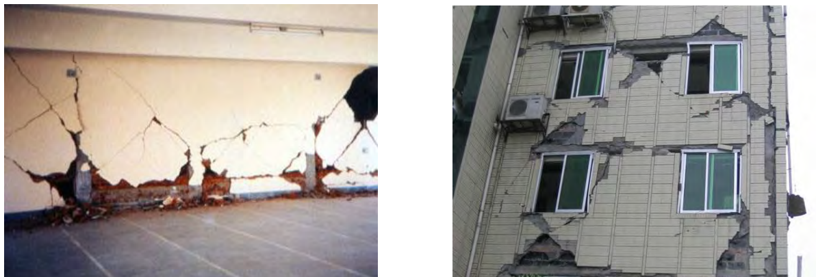
Figure 2.4 The filler wall damage
