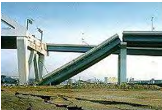
Figure 1.3 Bridge damaged in Hanshin earthquake
