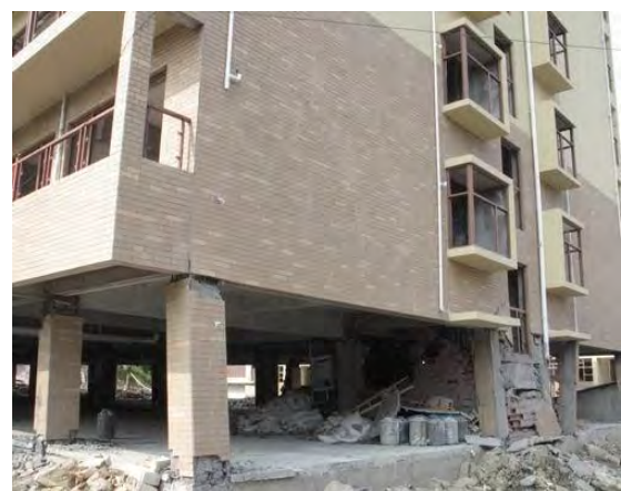
Figure 2.2 Example of collapse of the underlying framework
