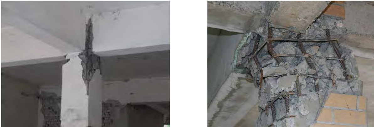
Figure 2.3 The extremity of column damage in the earthquake.
