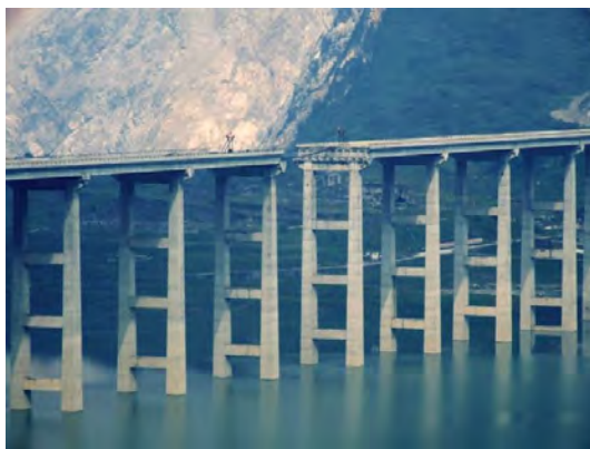
Figure 1.1 Miaoziping Bridge damaged in 2008 earthquake
