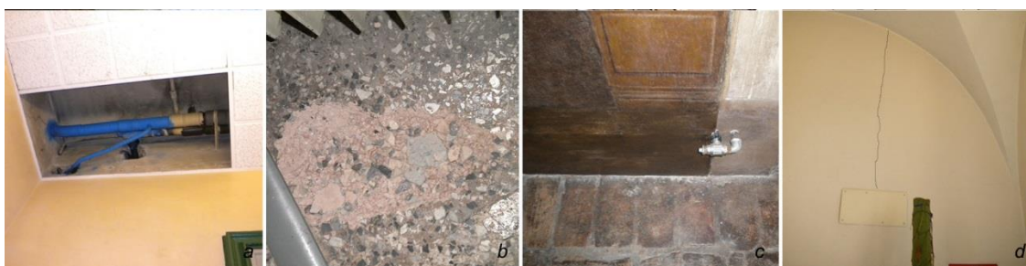
Figura 7.48: degrading promoted by the realization of plants: a) degradation of the ceiling in Ala Moschini ; b) disintegration of the Venetian terrazzo in the Sala del Consiglio ; c) damage to the frescoes in the Sala dei Nodari ; d) cracks in the plaster in correspondence of the traces of the electrical plant.
