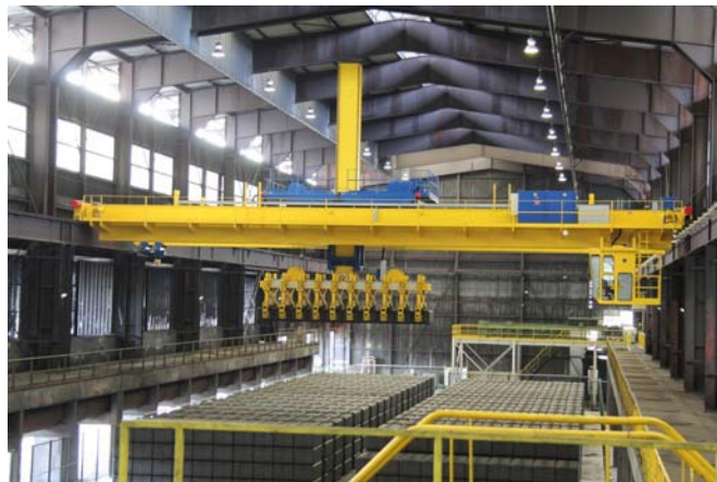
Figure 2.6: Carbon anode plant, anode rodding area
