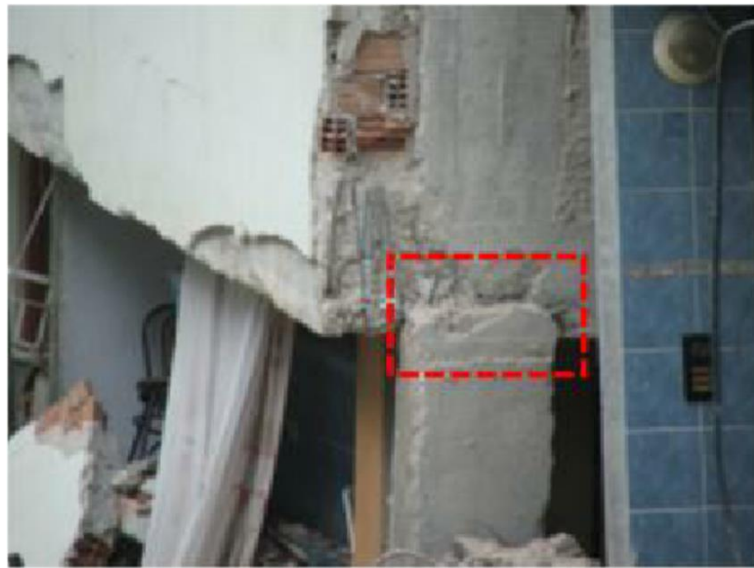
Figure 1.12. Exemple of failure cause by inadequate steel reinforcement (Adem Dogangun 2013)
