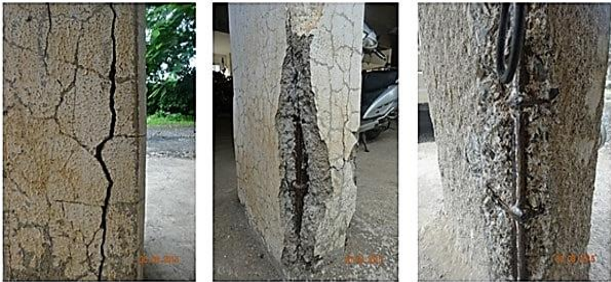
Figure 1.17. Poor concrete quality failure (Gopal Mishra, 2016)
