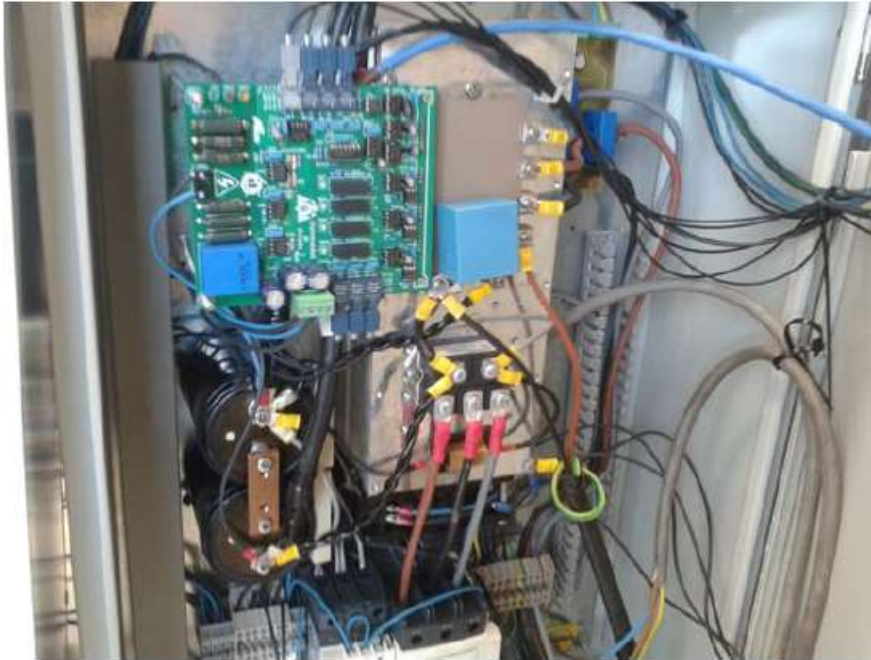
Figure 4.6 - Rectifier and inverted connected to the IM.
