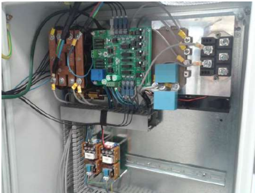
Figure 4.7 - Inverter connected to the IPM synchronous machine.
