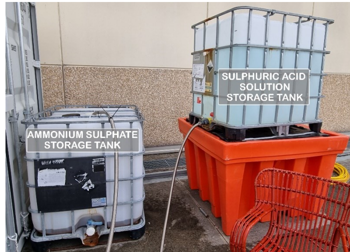
Figure 2.6: Sulphuric acid solution (scrubbing solution) and ammonium sulphate solution (final product) storage tanks
