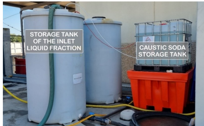
Figure 2.3: Inlet liquid fraction and caustic soda storage tanks
