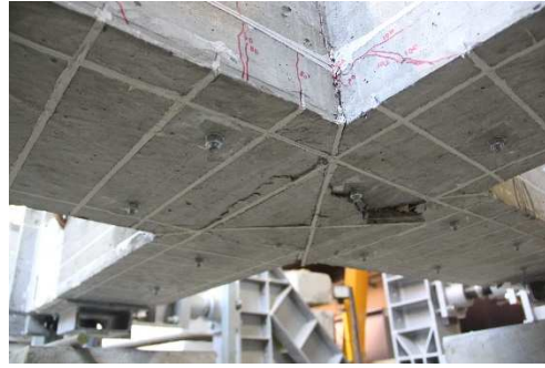
Figure 4.22 – Crack on the bottom surface, JPB joint
