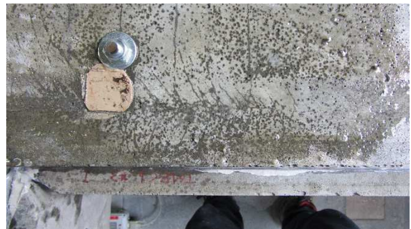
Figure 4.14 – Micro-cracks in SHCC panel along longitudinal carbon laminate location
