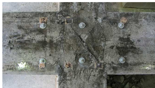
Figure 4.7 – Diagonal cracks in the joint region
