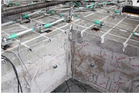
Figure 4.18 – Crack on the lateral surface, JPA-3
