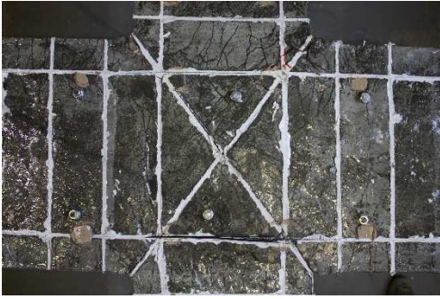
Figure 4.21 – Crack on the top surface, JPB joint
