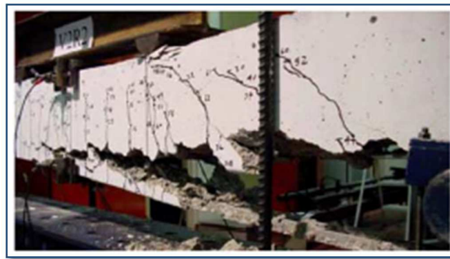
Figure 2.14 – NSM system, detachment of concrete layer [16]
