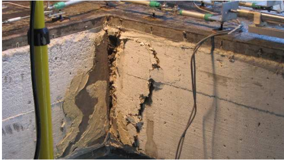
Figure 4.8 - Detachment of the old concrete cover
