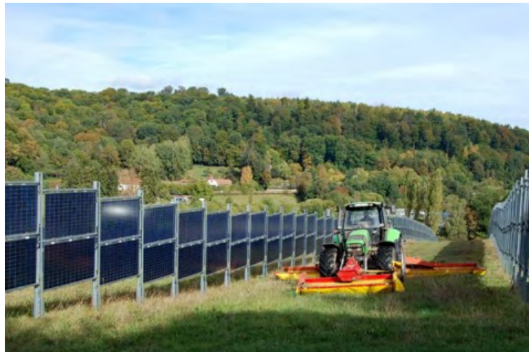
Picture 8 The vertical solar system that combines bifacial modules (© Next2Sun GmbH).
